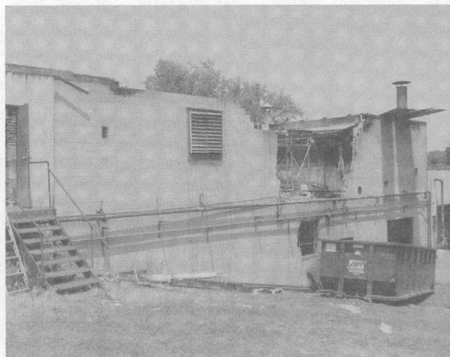
East outside wall in area where fire started
