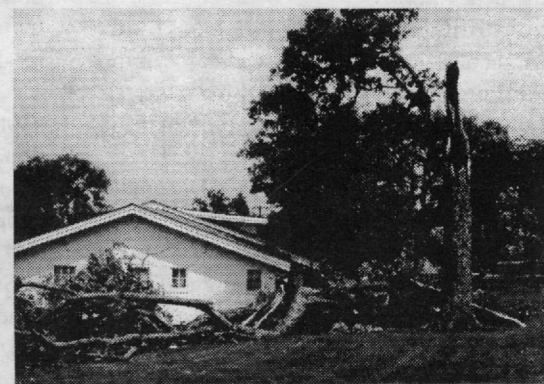
Storm damage, front.
