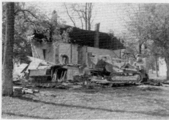
One of four small cottages by Williams Hall about to be demolished.
