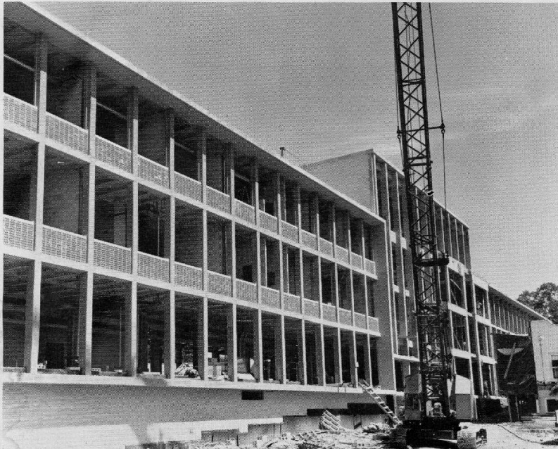
180-bed wing of Madison hospital under construction, showing progress on the three floors and boiler room at top. This wing is scheduled to open early in 1965.
